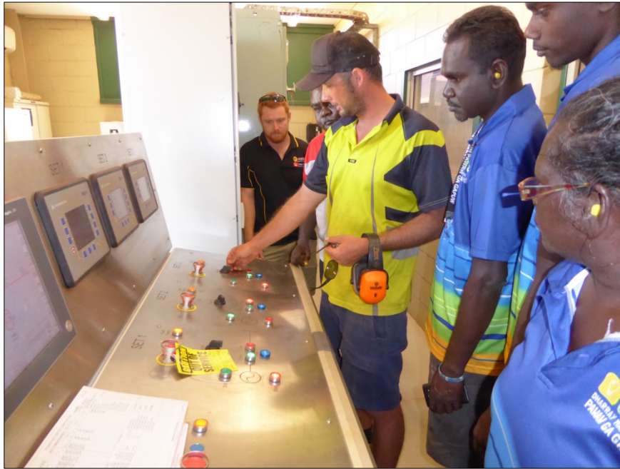
Site visit to the power station as part of the energy training
