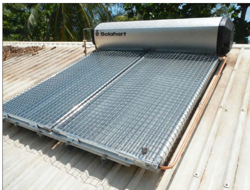
Solar hot water system installed as part of the project
