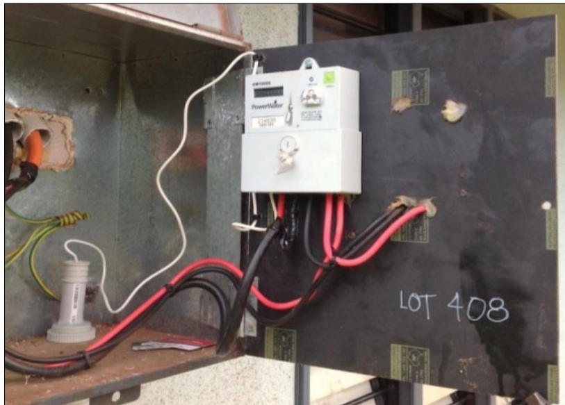
EM1000 and Taggle unit installed behind a typical meter board
