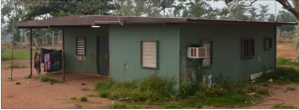
Beyond Economic Repair (BER) three-bedroom house, slab-on-ground with cement fibre composite wall cladding.
