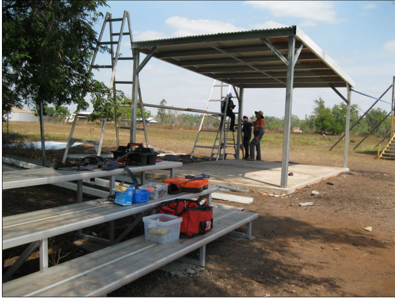
Construction of seating and shade at the Milingimbi sports oval by local RJCP workers
