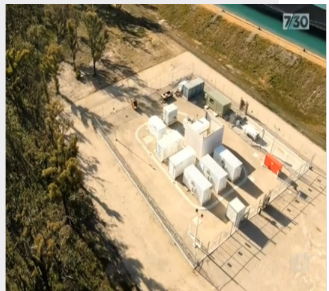
Mallacoota Emergency Power Supply Photo: ABC 7.30 report
